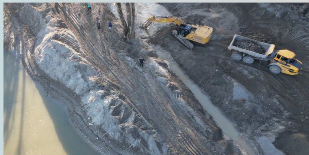
Figure 5: Construction works to remove soil and armour stones used for river bank fixation.
